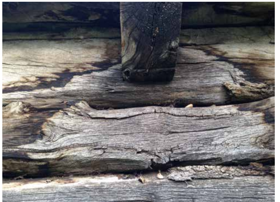
Current water damage on the exterior walls.
