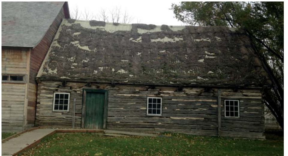
The Waldheim House in 2014 showing the deterioration of the roof and moisture damage of the log structure, particularly at the eaves.
