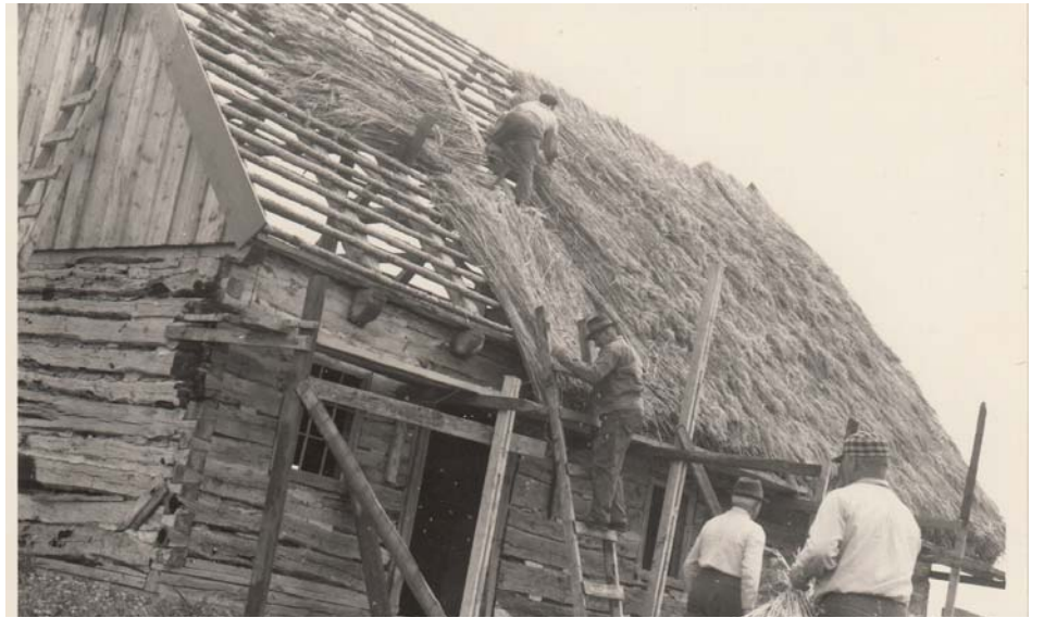
Thatching a new roof for the Waldheim House when it arrived at the museum, 1967.
