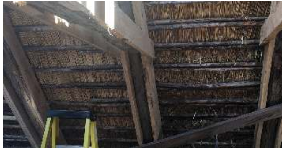
View of the underside of the roof in the attic as thatching is in progress.
